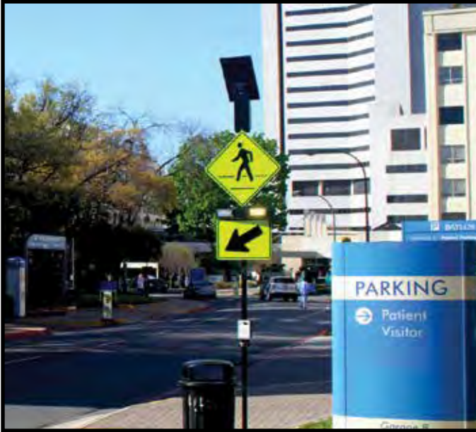
Solar Powered Rectangular Rapid Flashing Beacon
